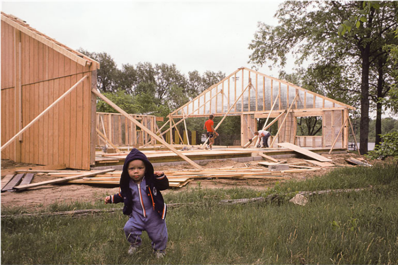
Russ Matero's son Lon seems more interested in what the photographer is doing than in the raising of the new sauna's walls.
