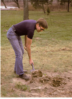
Harry Kansman, project manager, breaking ground for the new sauna building in the spring of 1982.
